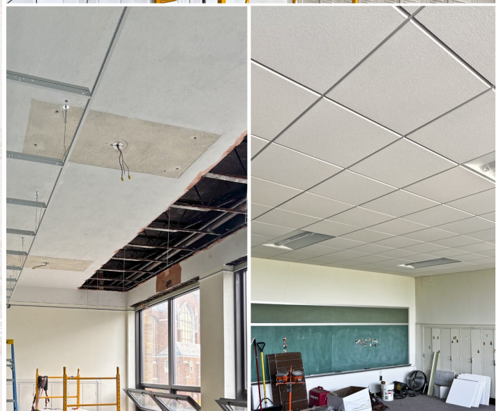
Work is nearing completion on the replacement of classroom ceilings, with modern LED lighting fixtures, in the Parish Center.
